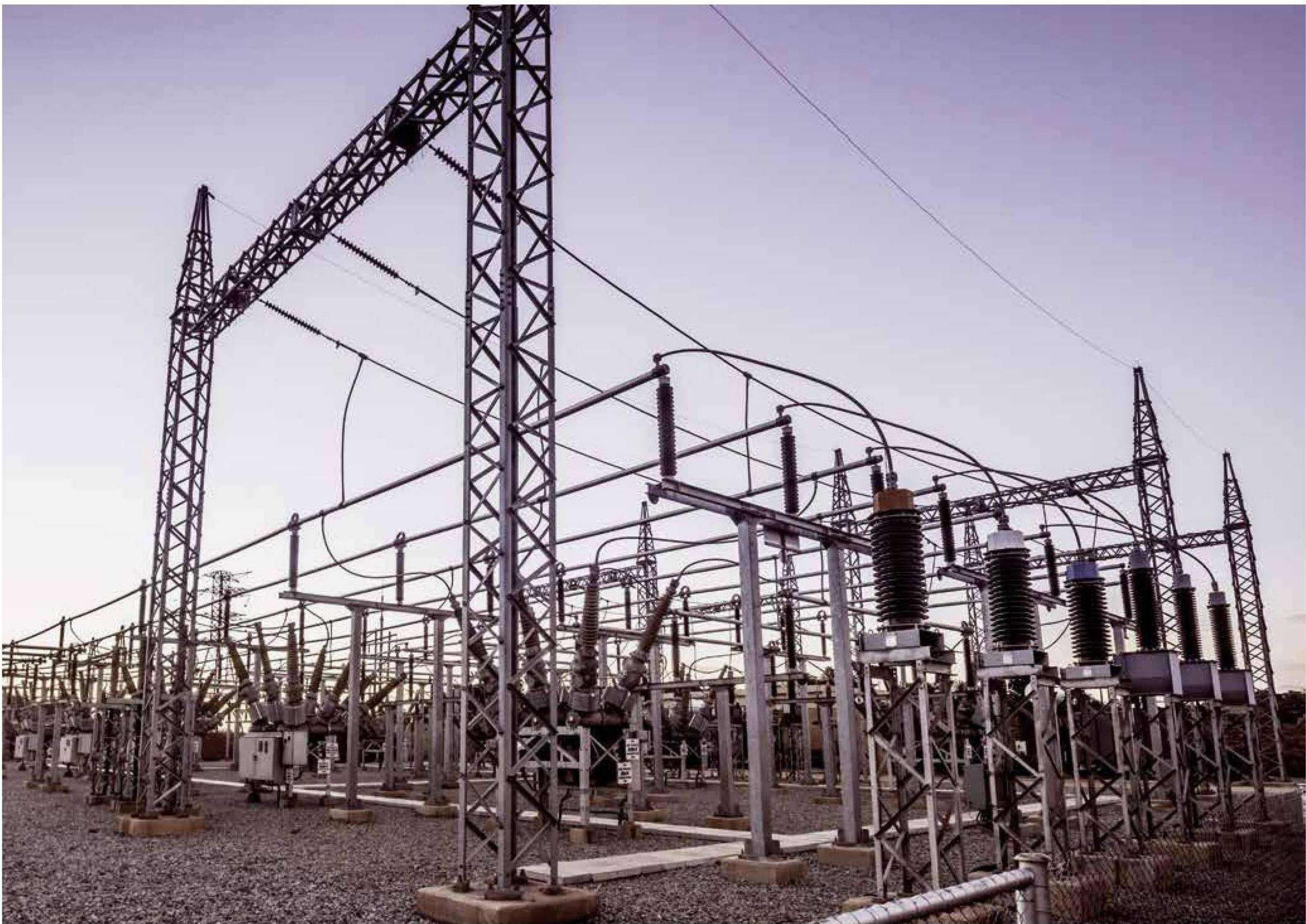
THE GOAL IN SOUTH AFRICA IS AN INTELLIGENT, MULTI-DIRECTIONAL POWER GRID THAT CAN BALANCE VARIABLE INPUTS FROM WIND AND SOLAR POWER PLANTS IN REAL TIME
