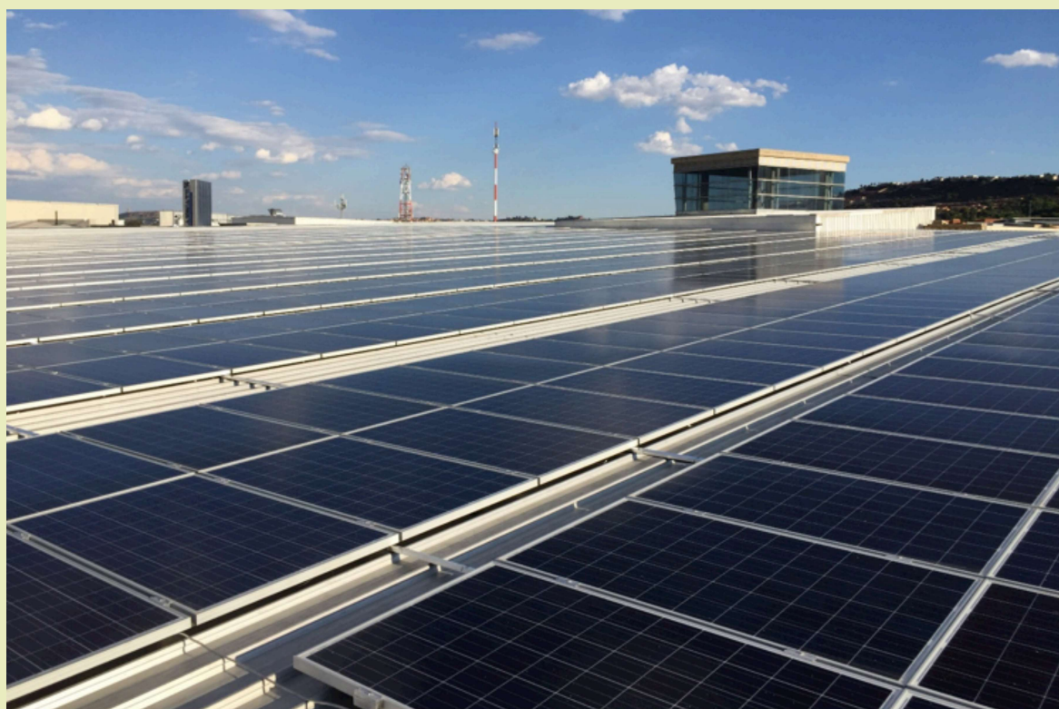
Figure 24: Clearwater Mall PV arrays
