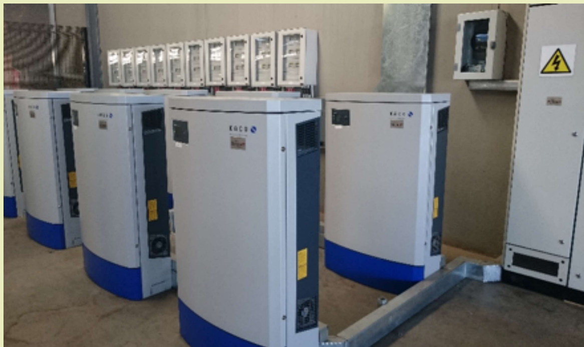
Figure 23: Clearwater Mall PV system inverter bank
