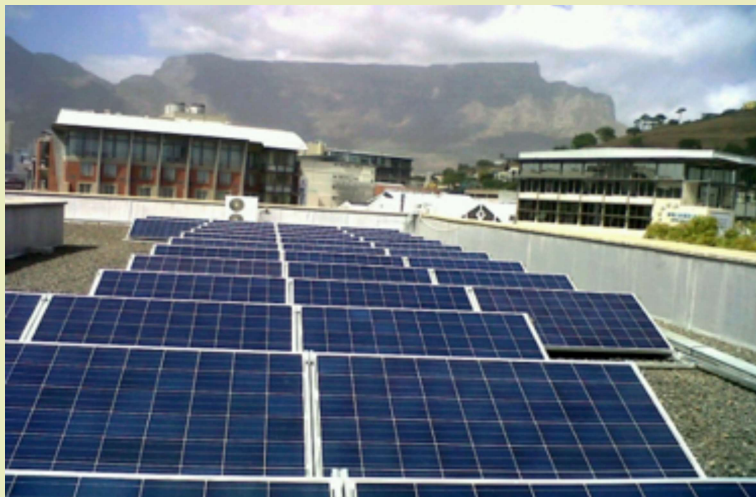
Figure 24: The PV array on the Gallows Hill roof
