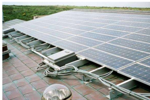
Sloped Roof mounted PV array, mechanically fastened 12
