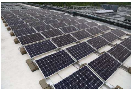
Roof mounted tilted PV array using ballasts 11
