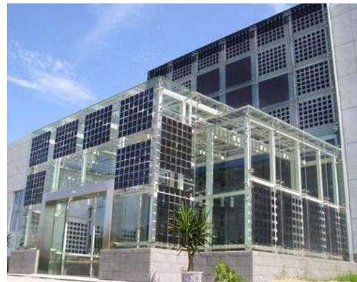
BIPV Window Application 8
