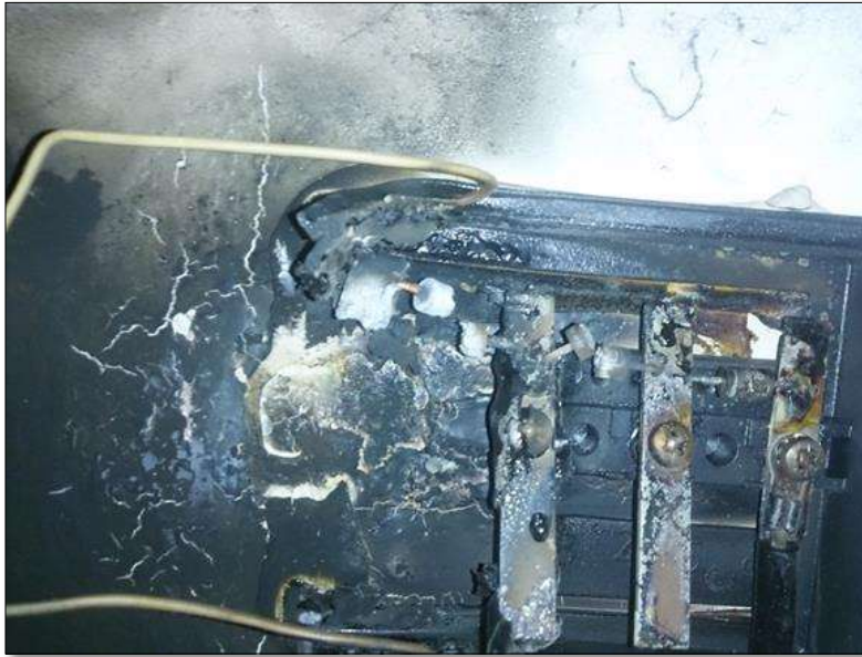
Figure 2-12: Bypass diode failure
